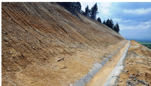
Figure 1 Soil slope with expressed erosion of the Highway Miladinovci – Shtip, R.N. Macedonia.
