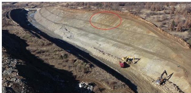
Figure 1 Aerial view of the cut: the studied area before the rockslide occurrence is marked with a red circle.
