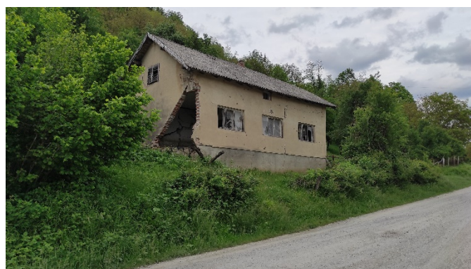
Figure 3. Abandoned and highly damaged masonry building above the unstable road section.
