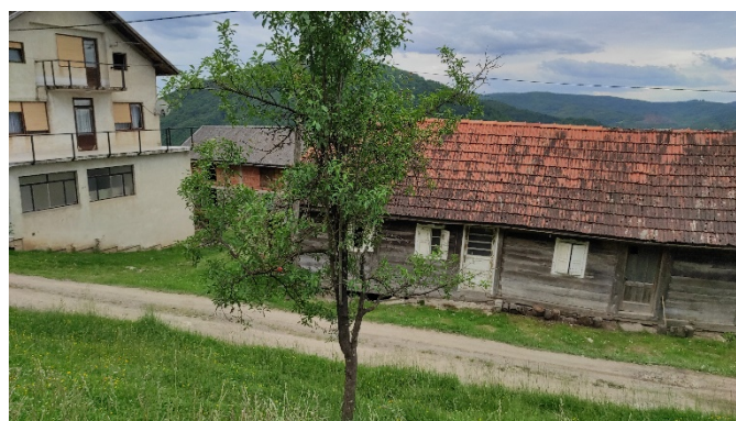
Figure 4. A damaged and leaned wooden shed below the unstable road embankment and an undamaged residential building with completely removed infrastructure.
