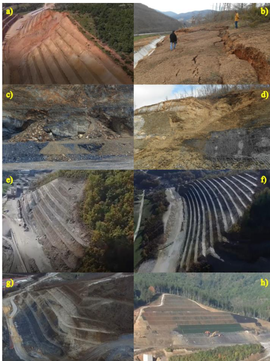
Figure 2. View of some of the representative cuts, along the route of the A2 motorway, section Kicevo – Ohrid: a) 3+400 – 3+961; b) 14+990 – 15+310 c) 11+745 – 12+140; d) 12+340 – 12+600; e) 13+327 – 13+576; f) 15+690 – 16+114; g) 13+770 – 14+000; h) 17+740 – 18+200.
