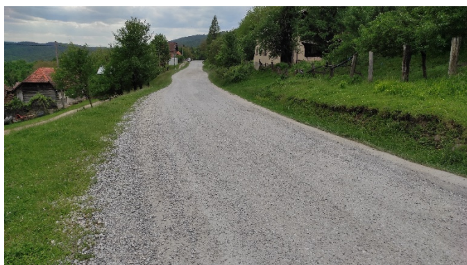
Figure 2. View towards the west on the unstable road section with the partly covered slide scarp along the northern edge of the road.
