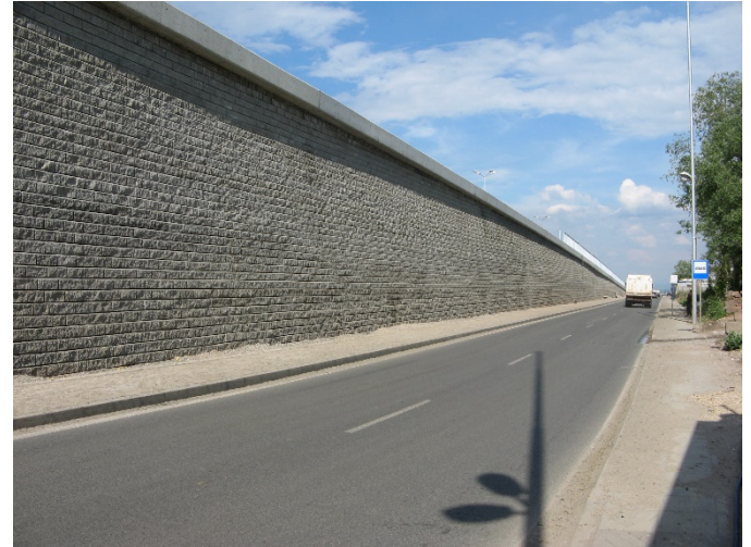
Figure 10 Fortrac Block GRS retaining wall in Sofia ring road project after earthquake in 2012 (Huesker).
