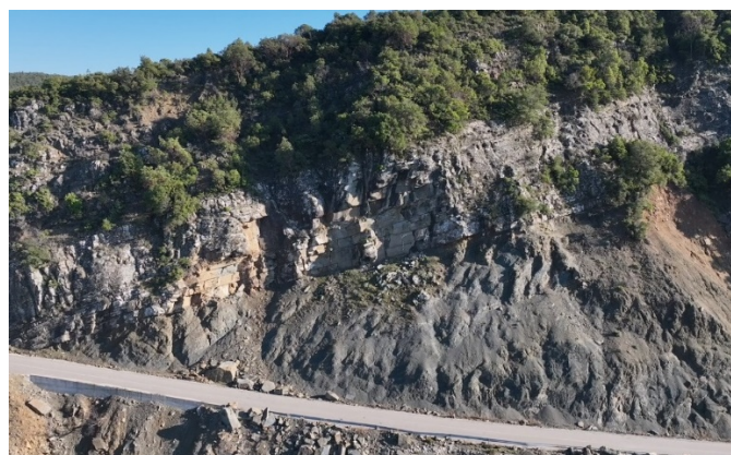
Figure 3 Significant rockfalls involving sandstone at the slope NE edge, directly above the provincial road. This activity is intensified by the undercutting of sandstone caused by the differential erosion of siltstone beneath it.
